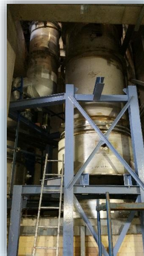
Recuperators in place
